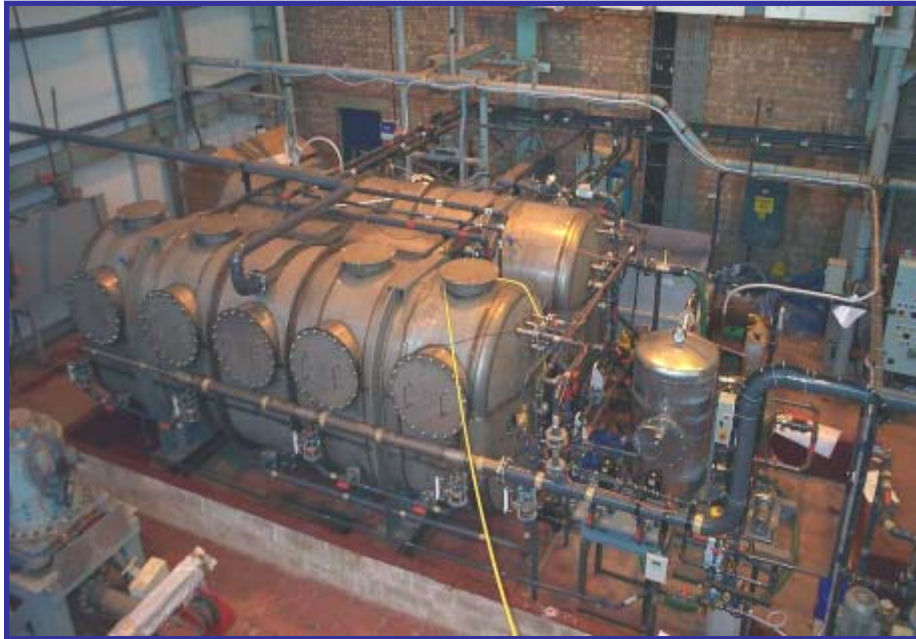
Development and retrofit of a Membrane Bio Reactor to HMS Grafton holding tanks
